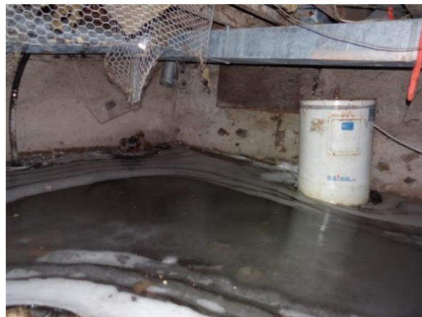
Plate 29: Detail of flooded basement.
