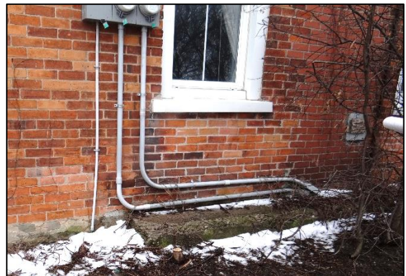
Plate 19: Detail of concrete feature along foundation and in-filled doorway (right), suggesting the location of a former veranda
