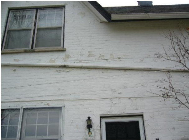
Plate 28: Enlarged window and door openings on north elevation with steel lintels and enlarged replacement windows (Cuming 2016).
