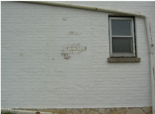
Plate 26: Original window on main floor of the west elevation was bricked-in and moved to the right (Cuming 2016).
