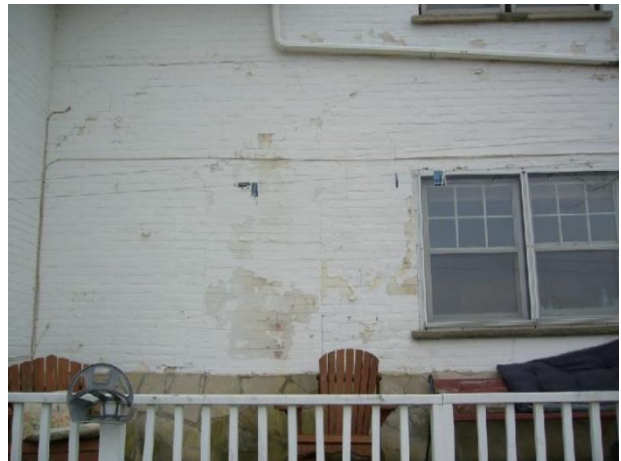
Plate 29: Bricked-in window opening to the left of the enlarged replacement windows and stone cladding at the base of the wall on north elevation of original structure (Cuming 2016).
