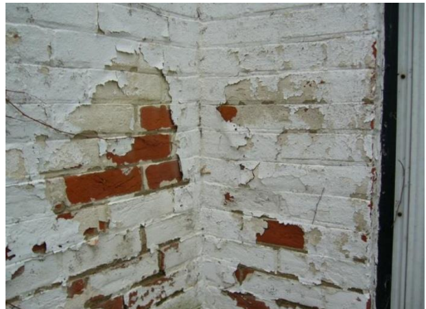
Plate 21: Detail of red brick cladding with cementitious finish and white paint on east elevation (Cumings 2016).
