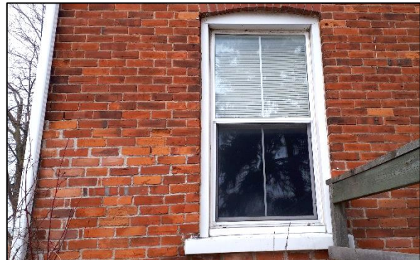
Plate 15: Detail vinyl window replacement on primary (east) elevation and repointed and spalling brick (left).
