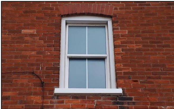
Plate 14: Detail of vinyl window replacement and (likely) vinyl or aluminum capped frame and sill. Brick deterioration is also observable.
