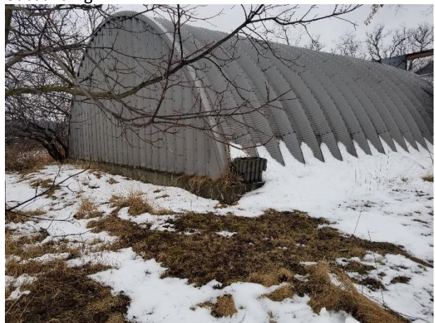
Plate 14: The east and south elevations of the drive shed, concrete pad foundation is visible
