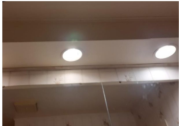
Plate 35: Drywall ceiling, vanity lighting, and wallpaper in the washroom (provided by owner).
