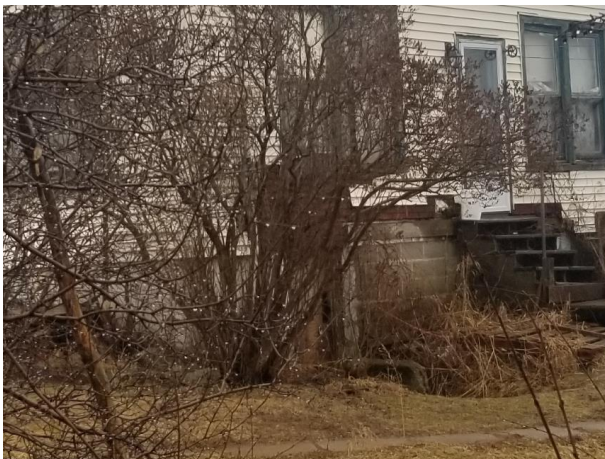
Plate 11: West portion of the south elevation with door leading to basement on the west of the main entrance, looking northeast.
