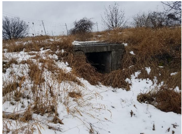
Plate 2: Cement box culvert under the driveway
