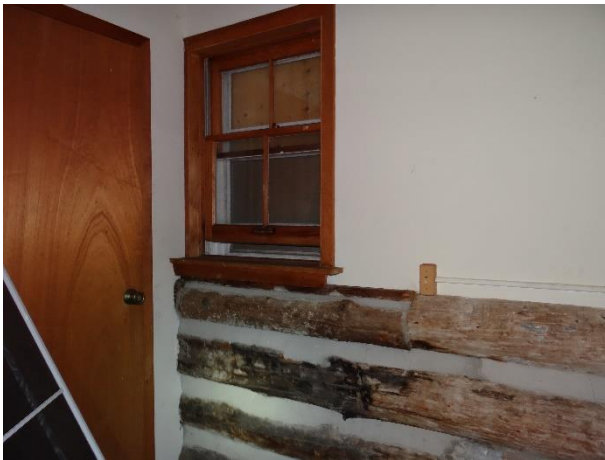
Plate 16: Detail of the logs and window on east wall of the hallway, log house second floor
